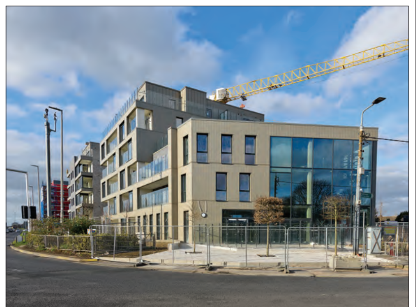
CONSTRUCTION: The Palmerstown Gate development at the former Vincent L Byrne site
