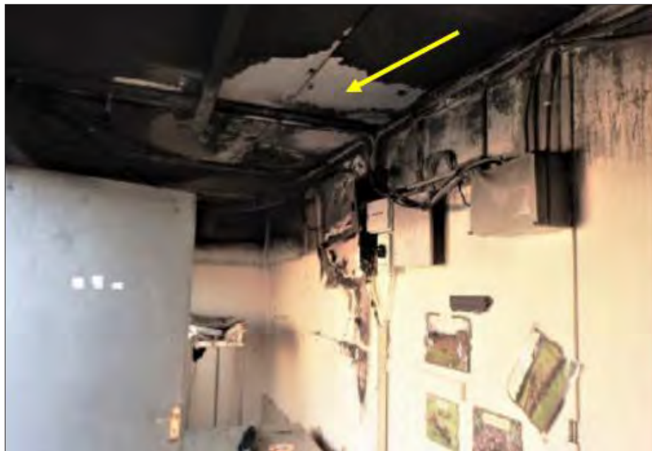
Entrance hall to the unit, now gutted from Electrical Fire damage.
