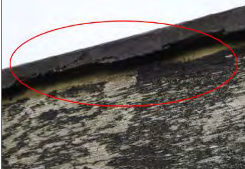
DISGRACE: Erosion of the felt membrane
