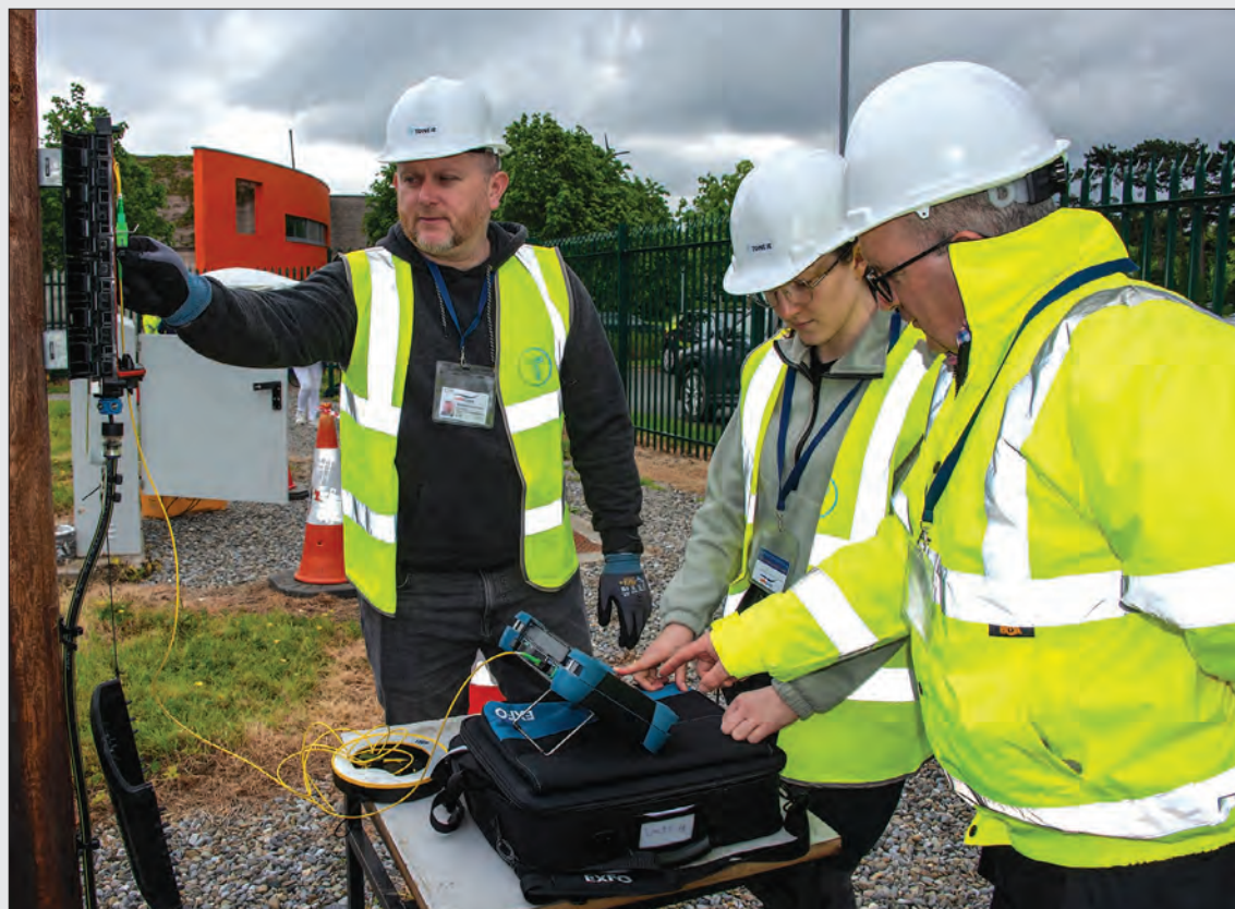
BEACON: Telecommunications and Data Network Engineering Apprenticeship students and lecturers demonstrate network installation outdoor training site on TU Dublin's Tallaght campus
